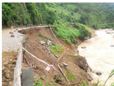
Negative talus or riverbank erosion
