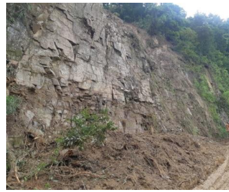
b. Debris and soil at MCC10
