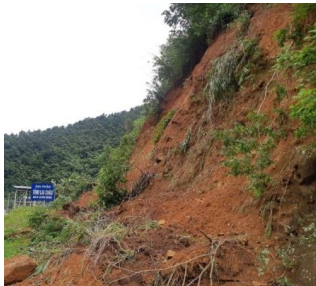
a. Debris fall at MCC01
