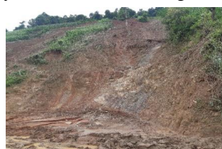
b. Soil flow at MCC24
