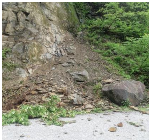
a. Debris fall at MCC02
