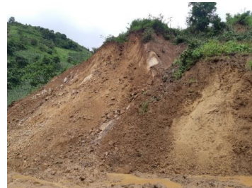
a. Debris and soil at MCC27
