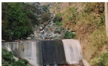
Figure 4. Water from Ma Le cave system flowing into Seo Ho stream in the dry seasons reaches 120 l/s
